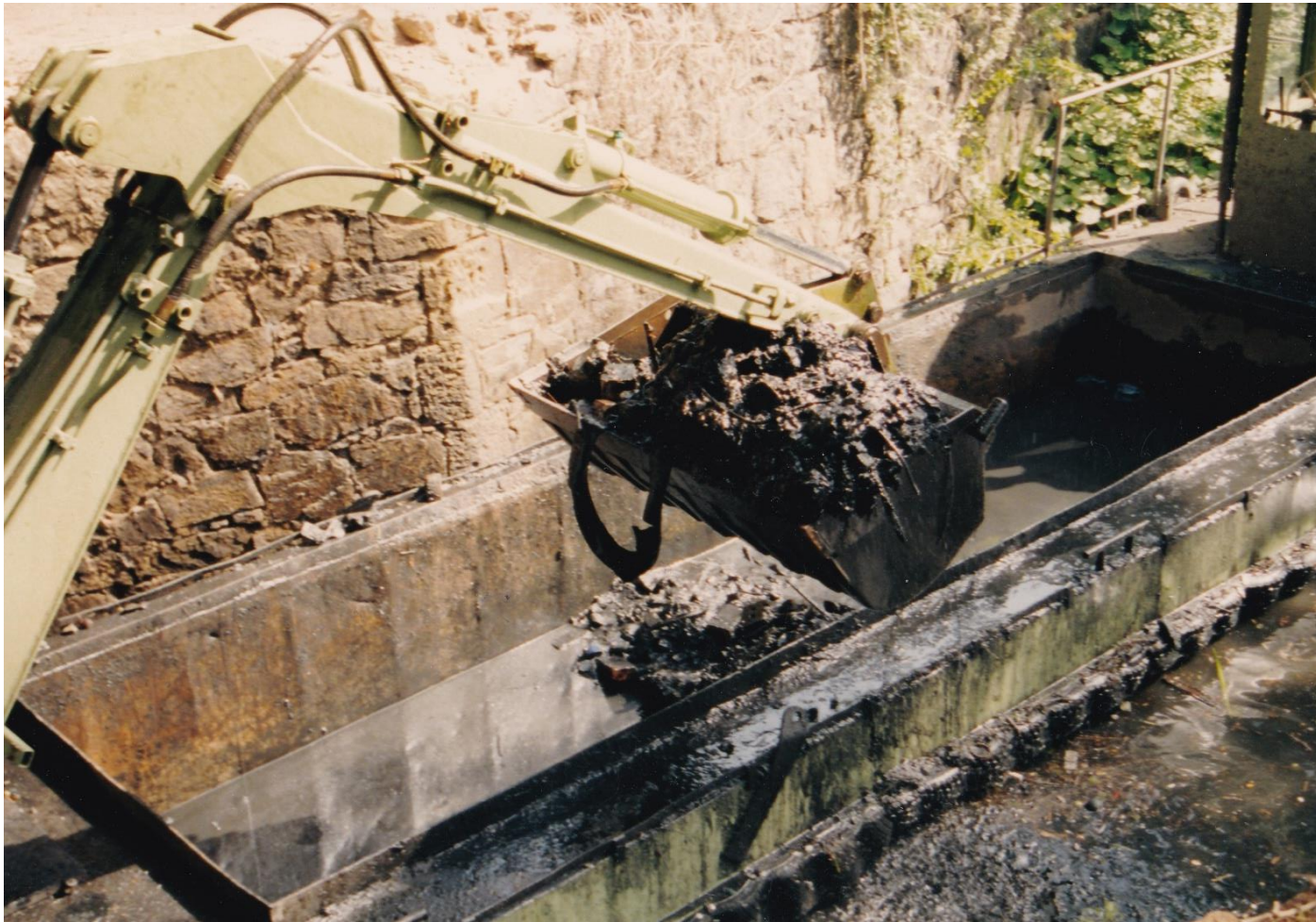
Figure 4: Desilting of the Karl Heine Canal by means of a floating barge and excavator
